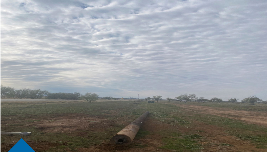
Completed the removal of the overhead utility poles at Access Business Park
